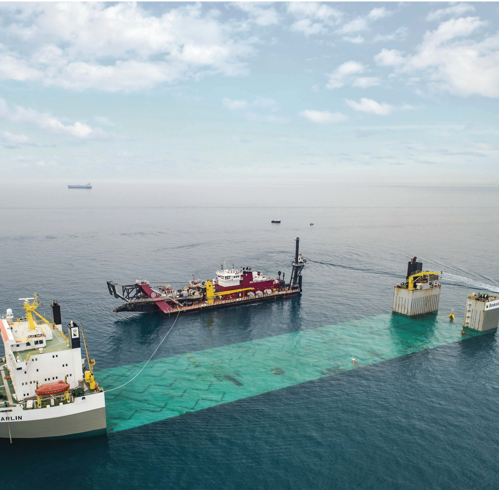
Dredge Ohio load out in Bahrain on a semi-submersible transport vessel in preparation for return to the U.S.
