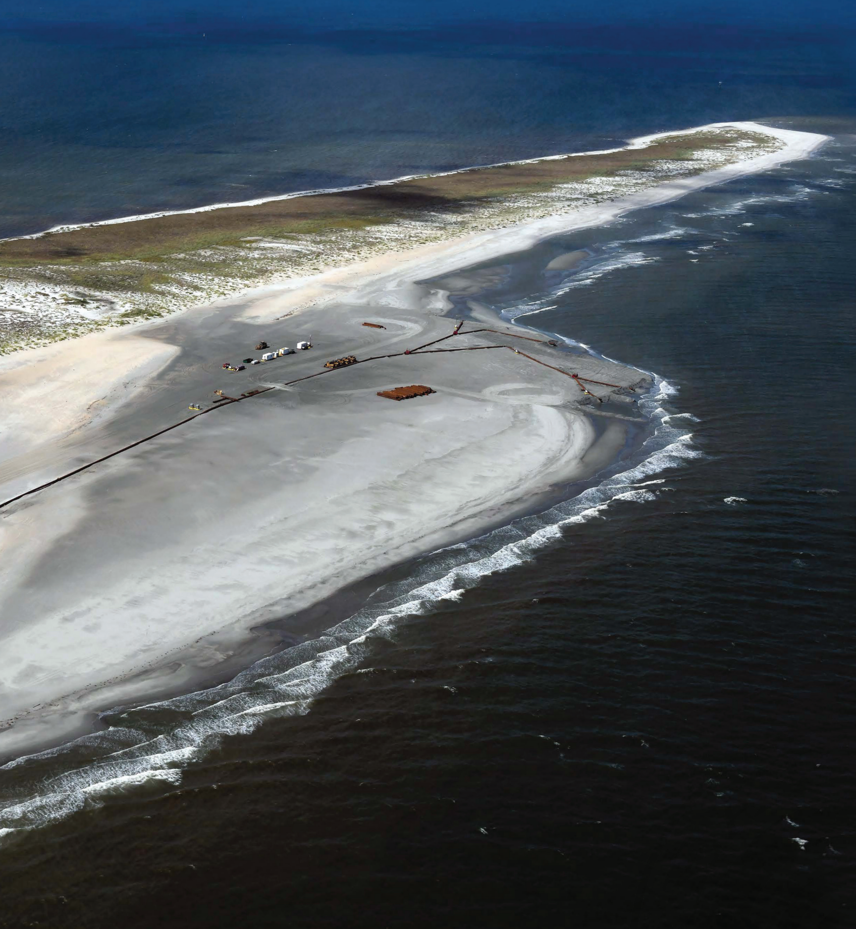
Photo Above: Mississippi Coastal Improvements Program (MSCIP) Beach Nourishment Phase III. Gulfport / Biloxi, MS
